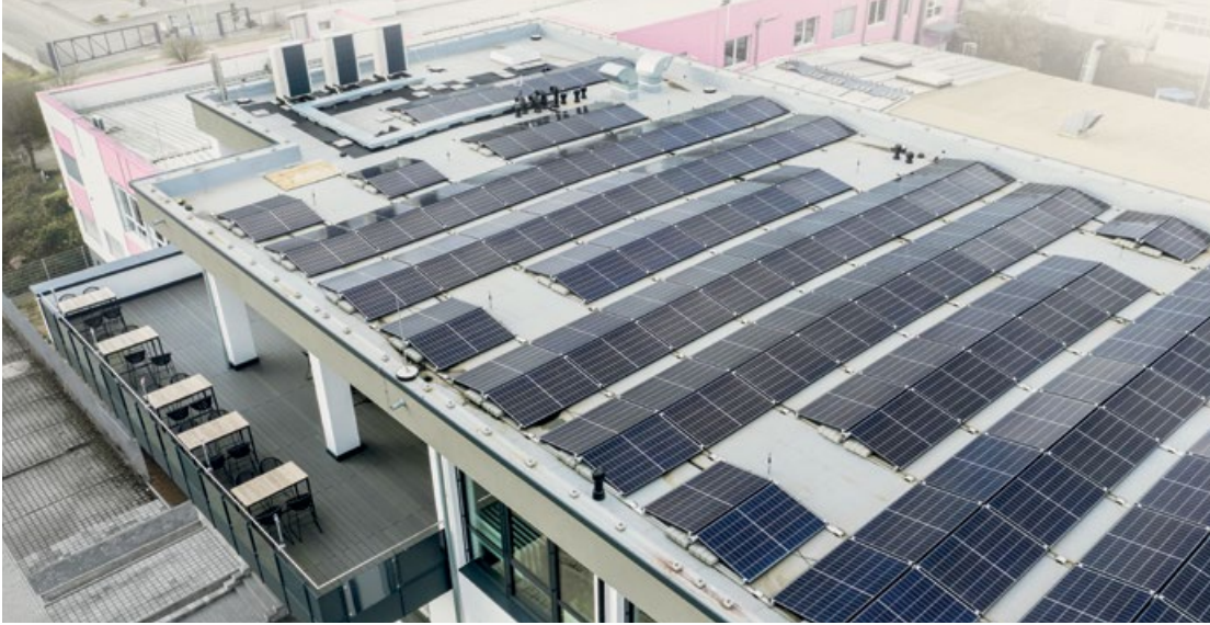
Photovoltaic system on building/plant 3B
